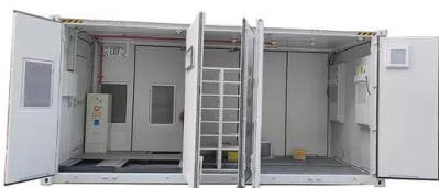
1075KW HH ESS
