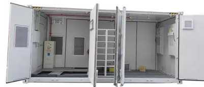
1075KW HH ESS
