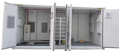
1075KW HH ESS
