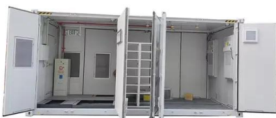
1075KW HH ESS
